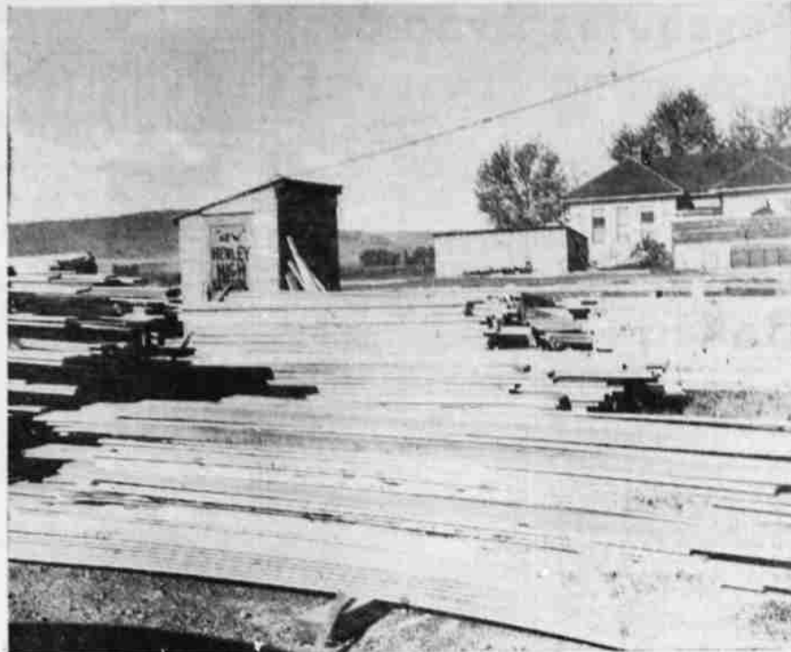
CONSTRUCTION SCENE—Work is getting under way at the new Henley high school building, one of the summer's major construction projects here. This picture was made Wednesday at the scene of activity on the Merrill road, Oregon 39.
