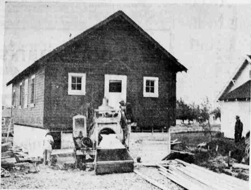
Former schoolhouse undergoing remodeling at Lakeview for new youth center. At far right is Andy Redmond, Lakeview, who is doing the work.
