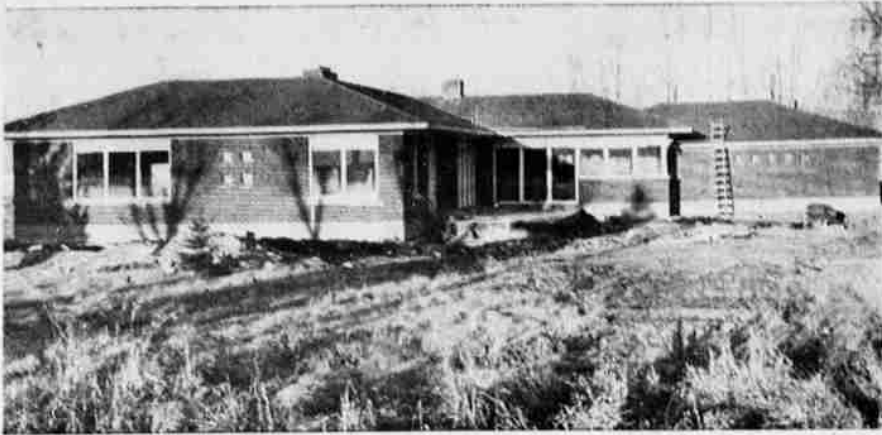
This house, about two-thirds completed, is located on the Alturas highway out of Tulelake. M. L. Sutton is the owner.
