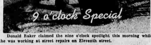
Donald Baker claimed the nine o'clock spotlight this morning while he was working at street repairs on Eleventh street.
