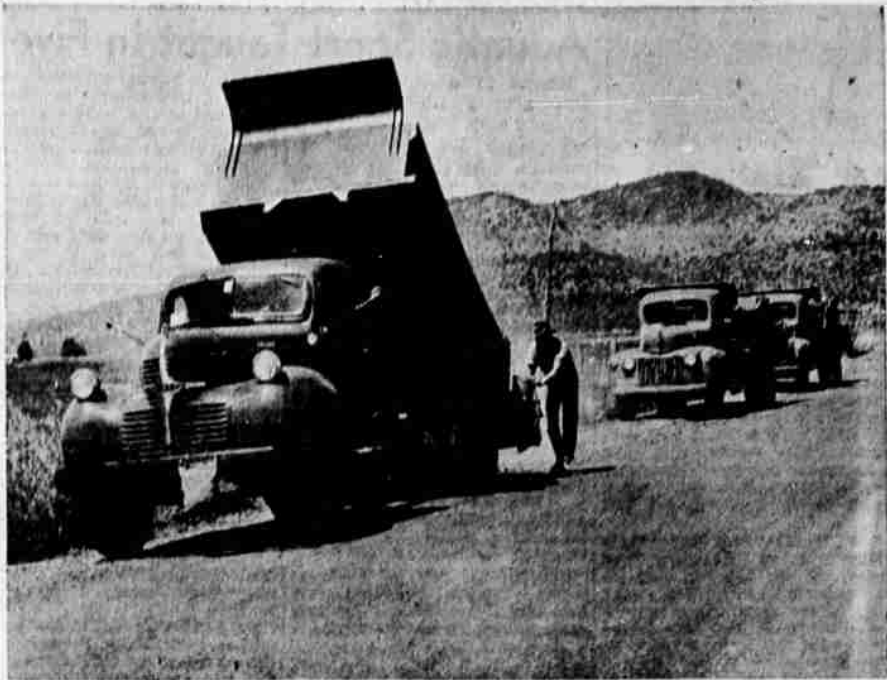
Part of the summer construction work of the Klamath county highway department is the surfacing of the Poe Valley road. This picture, taken by Herald and News Photographer Wes Guderian, shows county dump trucks at work.
