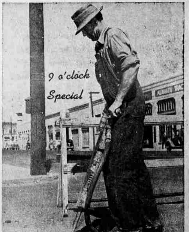
An early morning noisemaker caught by the nine o'clock photos is R. A. Meredith with his pneumatic hammer as he breaks out hunks of paving preparatory to patching on the corner of Main and Broad.
