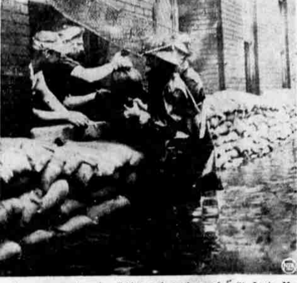
Emergency workers in oilskins and employees of a St. Louis, Mo., factory pile sand bags around the base of the building as water continues to rise. The building is five blocks from the Mississippi's shore at normal times.
