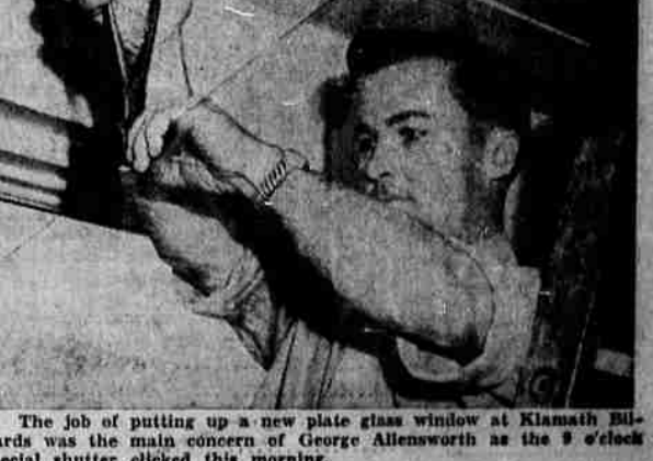
The job of putting up a new plate glass window at Klamath Billiards was the main concern of George Allensworth as the 9 o'clock special shutter elicited this morning.
