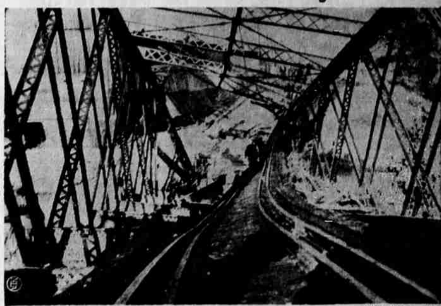
Twisted rails over this washed-out bridge are result of heavy rains which caused flood waters to burst through a dam at Rutland, Vt. (NEA Telephoto)
