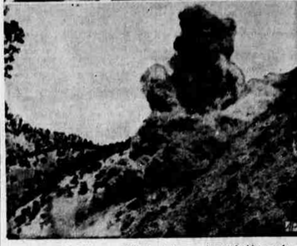
Governor Earl Warren (right, top) turns a key unlocking a charge of one ton of dynamite (below) to mark the start of construction of the $36,000,000 Pine Flat dam on the Kings river, 27 miles east of Fresno, Calif. At left is Col. E. H. Marks, retiring Pacific division engineer for the army corps of engineers.
