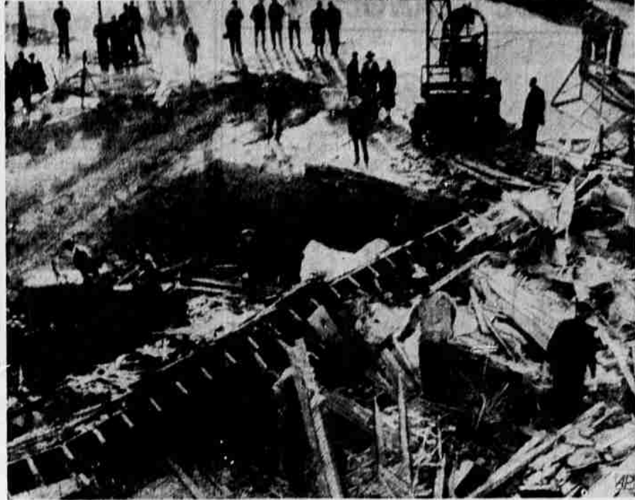
Rescue workers with machinery search for victims in the rubble of an apartment house-business building which collapsed into an adjacent excavation at Elko, Nev., killing three persons and injuring four others. —AP wirephoto.
