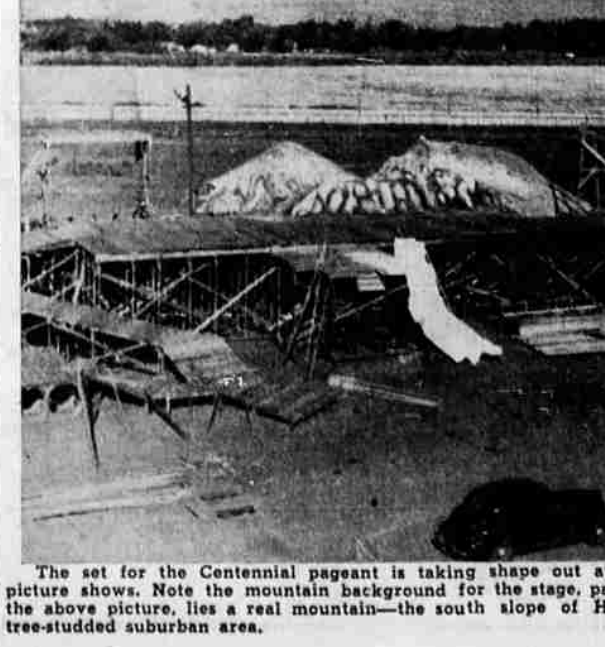
The set for the Centennial pageant is taking shape out at the county fairgrounds, as this picture shows. Note the mountain background for the stage, partially completed. Beyond that, in the above picture, lies a real mountain—the south slope of Hogback, and closer at hand the tree-studded suburban area.
