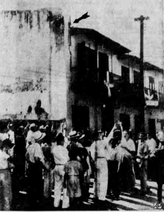
Members of the downtown crowd point to a crack (arrow) in a building in the downtown section of Ciudad Trujillo, Dominican Republic, left by the sharp earthquake felt the world around. Photo by Bob Glanders, Miami Daily News and flown to Miami. —AP wirephoto.
