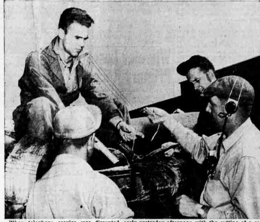
When telephone service was disrupted early yesterday afternoon with the cutting of a cable serving the south suburban area, workmen were faced with the terrific task of tagging 400 pairs of lines. Here some of the crew are matching the pairs. With back to the camera, James E. Weddell, and left to right, Don Reverman, Bob Haggerty, all of Medford, and Norm Smith, this city. The emergency crew was made up of three from Medford and three from Klamath Falls.
