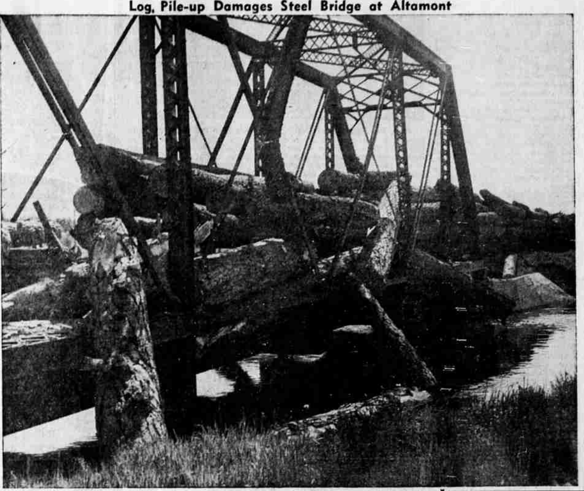
Log, Pile-up Damages Steel Bridge at Altamont
