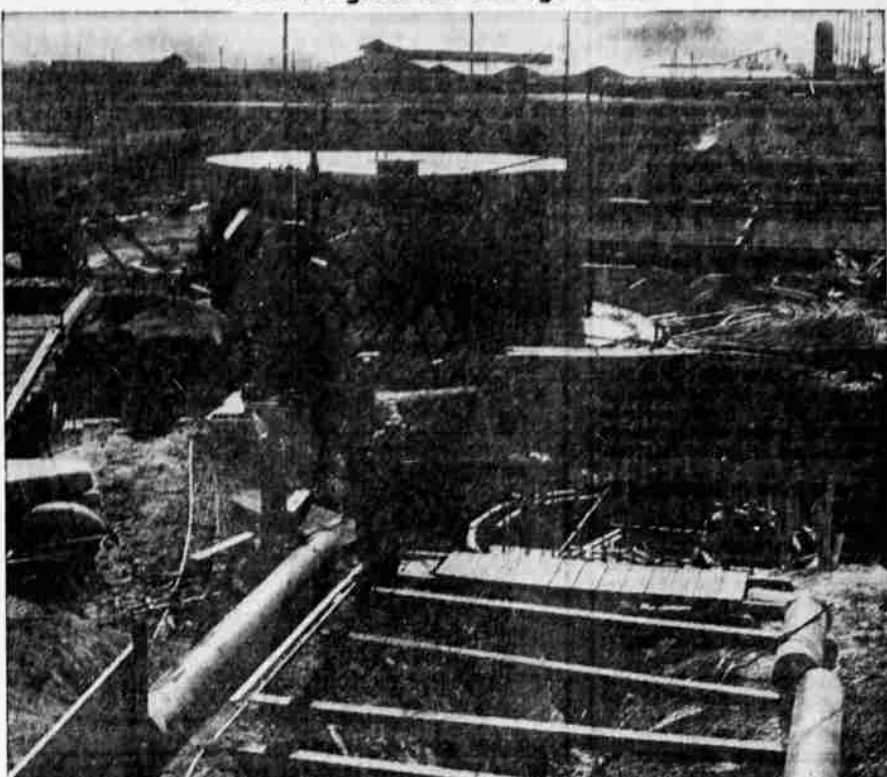
Work on the federal public housing sewage disposal plant, Shasta way and Owens, is progressing slowly because of a shortage of materials and slow delivery service. Shown above in the lower right hand corner is the round structure which is the beginning of a pump house. The round tank in the center is a two-story clarifier for sewage purification. Construction on the project began in mid-February.
