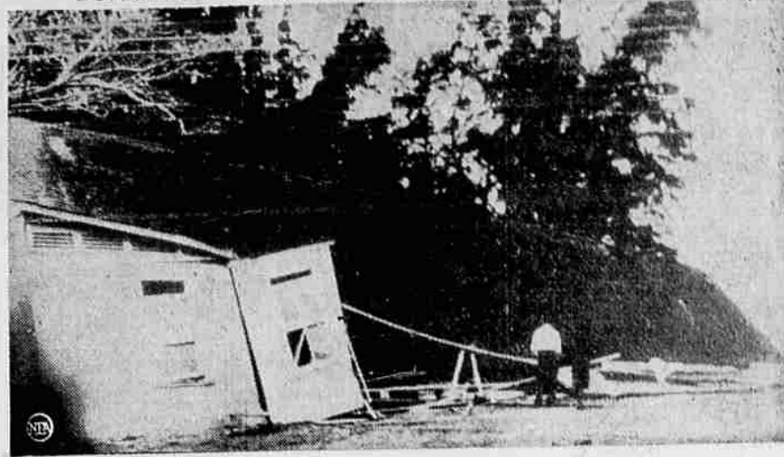
The worst tidal wave in the history of the Hawaiian Islands struck the islands leaving more than 10,000 homeless, 300 drowned or missing and causing millions of dollars worth of damage. Here is a home at Haliewa, Oahu, T. H., damaged by the wave as it struck. (NEA-Acme radio-telephoto from signal corps).
