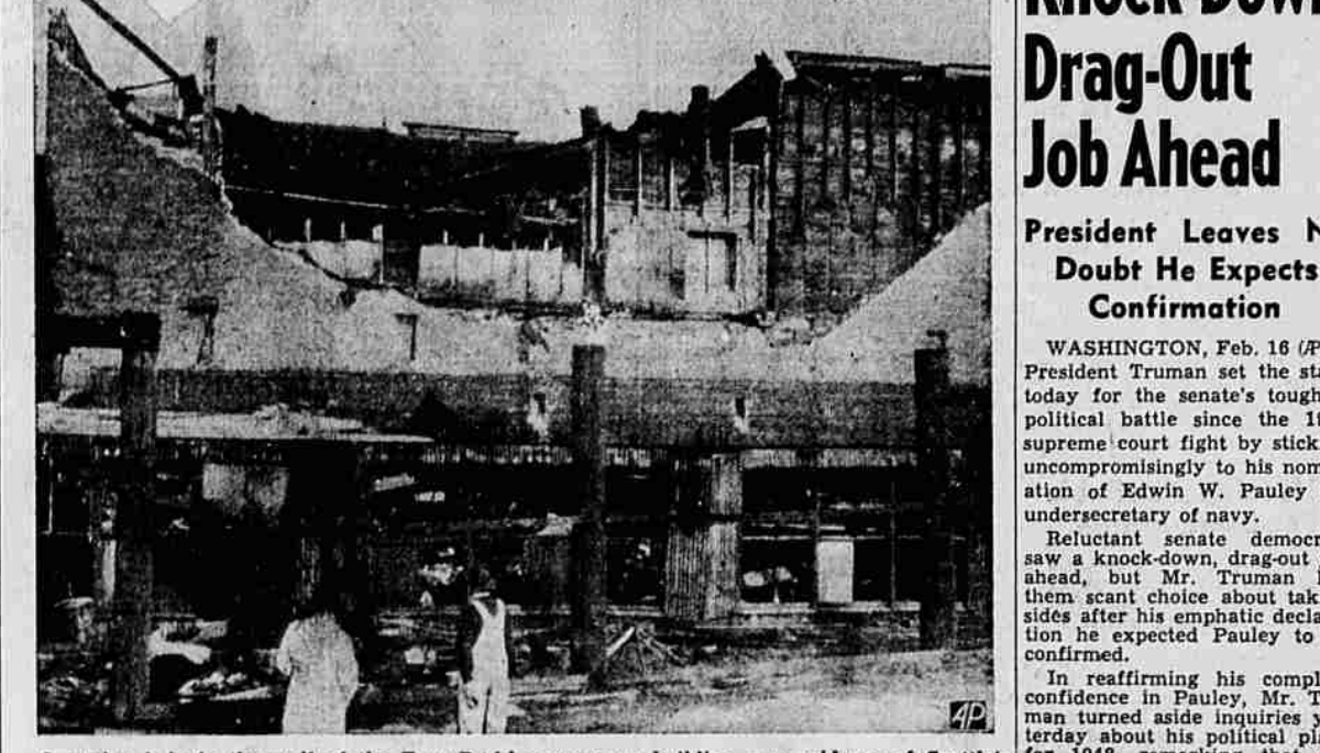
A gaping hole in the wall of the Frye Packing company building was evidence of Seattle's heavy earthquake. Bricks from an 80-foot section toppled on machine shop. —AP wirephoto.
