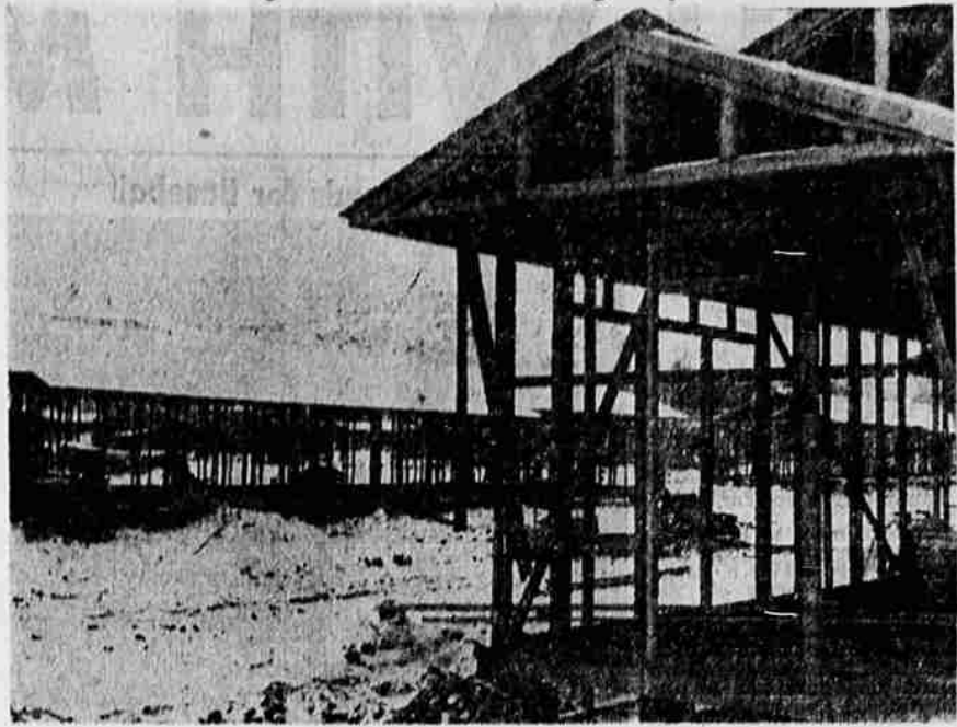
This picture indicates the progress being made on construction of an 80-unit housing project on Washburn way, on land previously held by the county school district. This row housing is being built for the use of families of military personnel.
