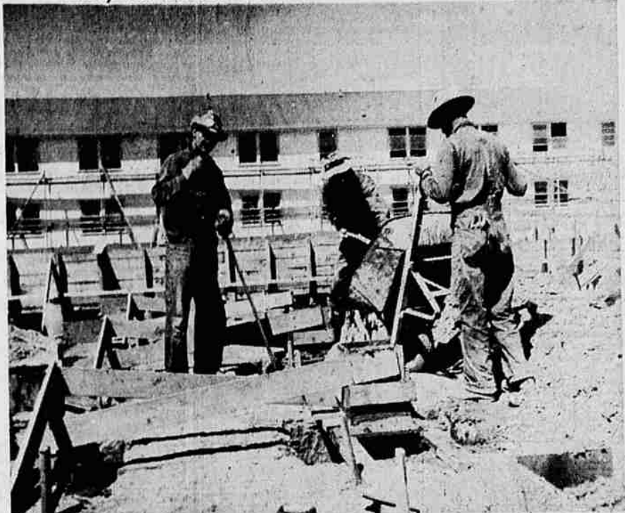
Under beautiful Klamath weather, construction activities at the naval air station have reached a new peak. With the pouring of footings for the officers’ club and subsistence building, contractors entered the last leg of the expansion program for officer housing. Shown in the background is the new type officers’ quarters, which are of stucco finish and light in color, in contrast to the drab green formerly used.
