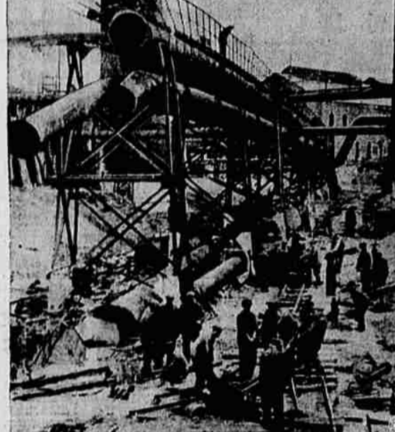
Although pretty busy with the war, Russians lose no time in rebuilding destroyed industrial installations. Photo above shows soviet workers at Yankiv reconstructing huge plant demolished by Germans before they fled from red army.
