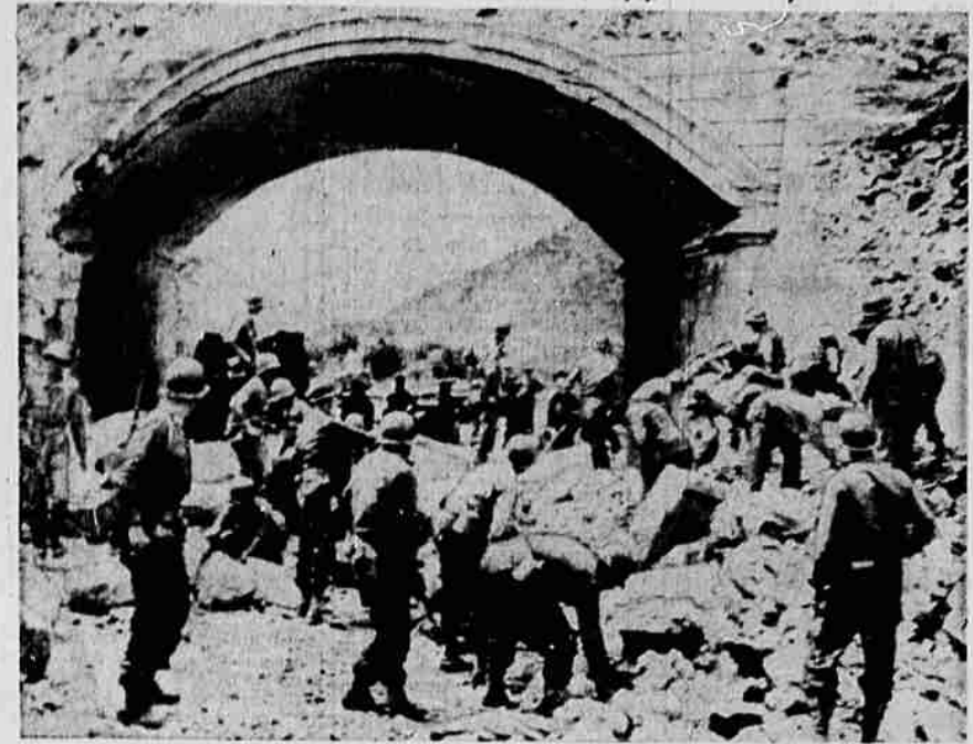
(NEA Radio Telephone Photo) After the capture of Itri, key town near the Italian coast, American engineers are shown as they cleared the Appian Way, important coastal road to Rome, along which Yanks have advanced to Terracina, half way to a junction with their comrades at Anzio. Signal Corps radio-telephone.
