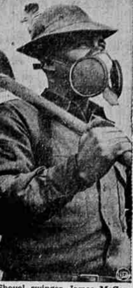
Shovel swinger James McCormack of Brooklyn, a U. S. private, wears dust mask when working along the road to Alaska.
