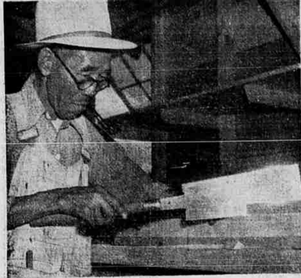
JAPANESE CABINET WORKER —Cabinet worker's saw, is expertly used by Jime Kabayashi, 62, on the interior construction of general store No. 2 at Tule lake war relocation authority center for evacuees of Japanese descent. Jime, prior to evacuation, had resided in Sacramento for 24 years and has been a carpenter for 42 years.
