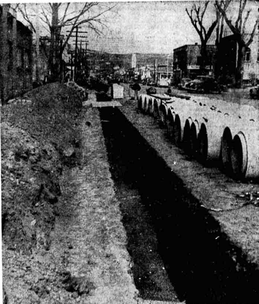
STREET CONSTRUCTION JOB —Klamath avenue scene shows construction of new storm sewers for which Klamath people voted millage year or two ago. WPA is helping on the job.
