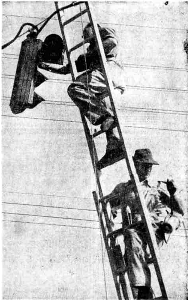
STOP AND GO —A long-awaited traffic improvement came in 1941. Picture shows workmen installing one of the new stop and go signals.
