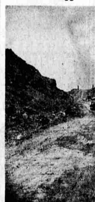
This picture shows heavy equipment at work on the rugged re-location construction on The Dalles-California highway just north of Klamath Falls.
