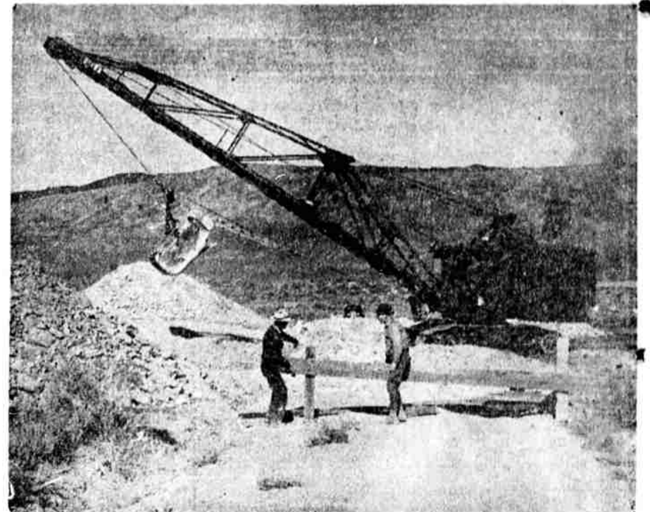
SUMP —The sump development was one of the "favored for 'forty" projects, prominently discussed at the beginning of the year, which actually got under way. Picture shows construction starting on an outlet canal on Lower Klamath lake.
