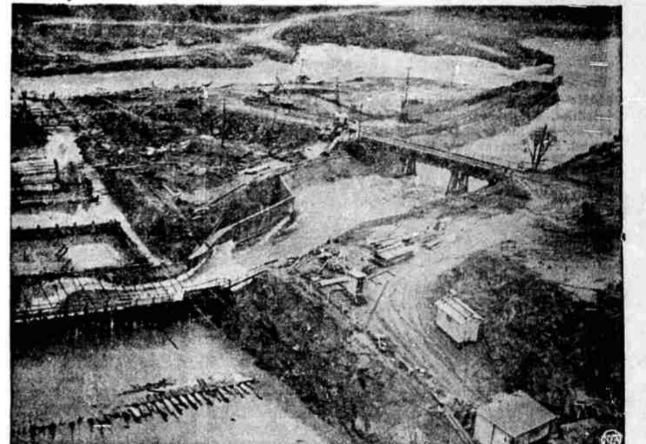
Heavy rains which fell over California incessantly for two weeks put a temporary halt to construction of Friant Dam, a portion of the Central Valley Water Project near Fresno. Here's a view of damage caused when the San Joaquin River went on a rampage, running an estimated 11,000 feet a second.
