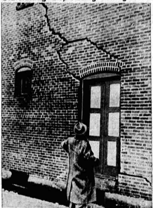
A resident of Shenandoah, Pa., looks at a widening crack in the city's railway depot, after cave-ins split the walls of homes and business places. The "sinking city" is built over old coal mines that honeycomb the mountain below town.
