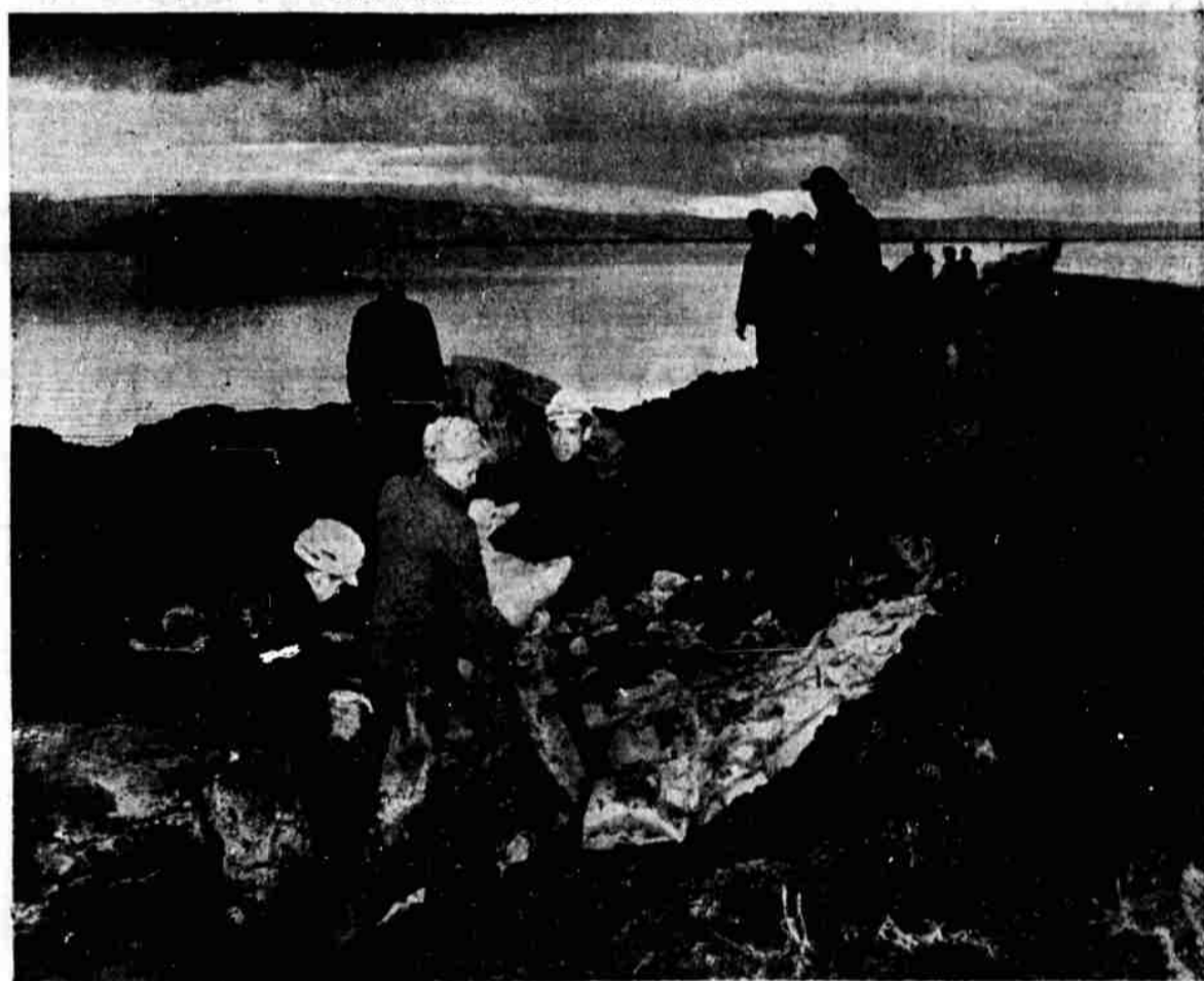
ATTACK AND DEFENSE—CCC boys from Tulelake camp strengthening a dike. The open water seen in the picture is highly dangerous to such protective structures, for there is nothing to break the wind and wave action.
