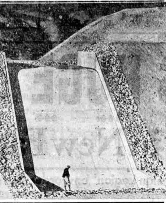
Several wash intakes like the one pictured will protect the banks of the All-American Canal from flood action—despite the fact that the canal crosses a desert region. The intakes are to take care of cloudbursts. The All-American, to be America's largest irrigation canal, will water large areas in California's Imperial Valley.
