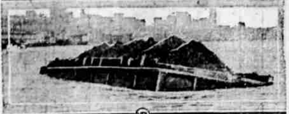
These pictures show how the mountain is being moved from the heart of Seattle. Above, one of the steam shovels and endless conveyor belt which leads to the water front where the dirt is taken out on scows and dumped, as shown below.
