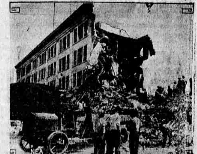
Santa Barbara is hard at work repairing the devastation wrought by her earthquake. This picture shows workmen busy on the ruins of the San Marco building, which was one of the largest in the city.
