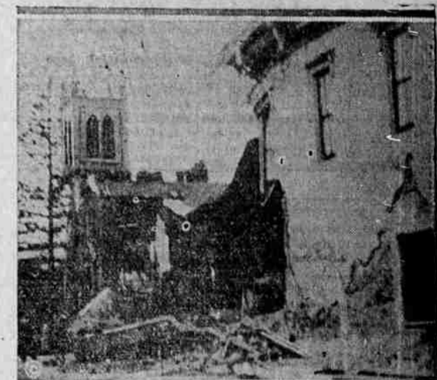
Santa Barbara's earthquake partially demolished its famous mission: this photograph shows how the Catholic church, standing alongside of the Knights of Pythias hall, was ruined.
