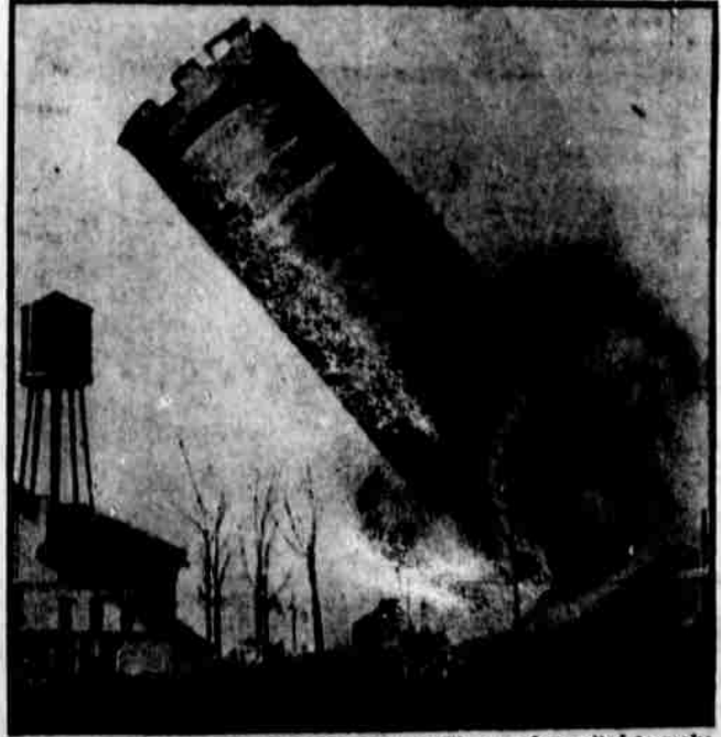
This 200-ton cement silo at Mooseheart, Ill., was dynamited to make way for a canal in honor of James J. Davis, founder of the Mooseheart home and sanctuary of labor. It will be dedicated next June by President Harding. A companion job, that's a real job.
