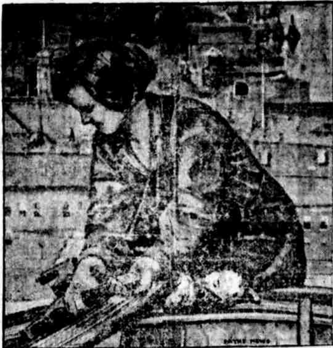
"Dizzy? Never!" says Mrs. Catherine Nelson. She's 300 feet up in the air, welding a bridge span at Kingston, N. Y. She sets $30 a day. Welding cables is her specialty.
