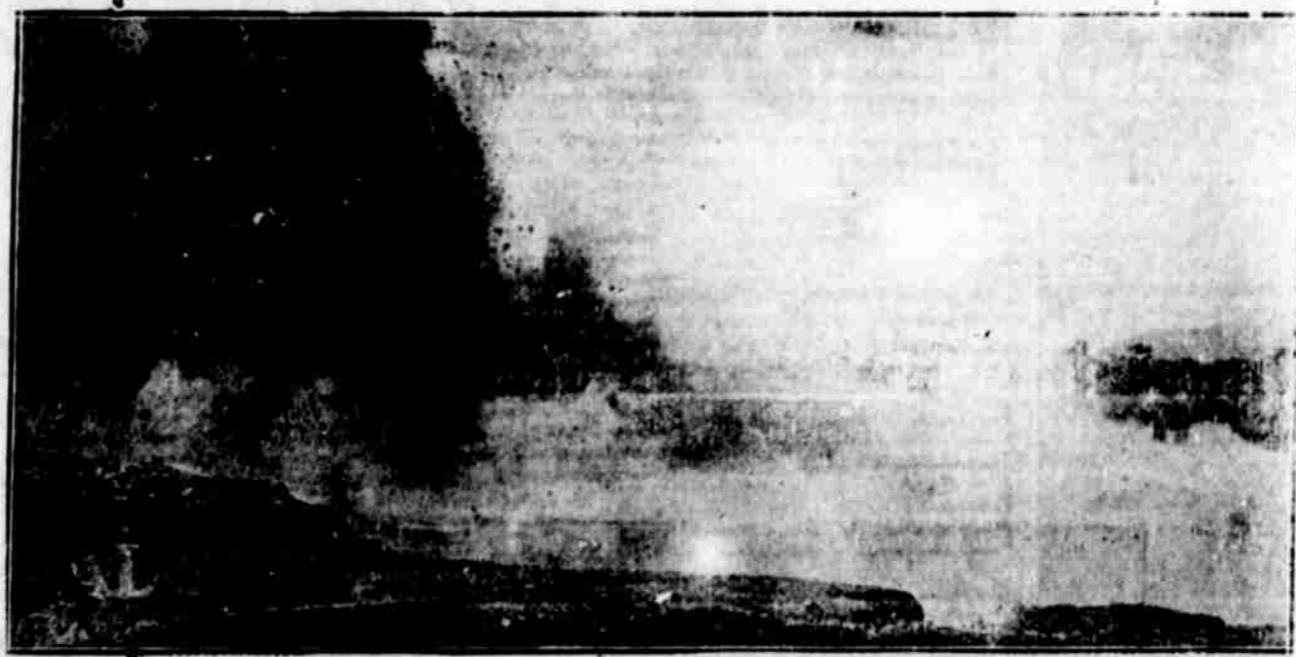
Twenty tons of dynamite were used by the engineers of the Panama canal to open it to the waters of the Pacific Ocean. They shot a blast on the dyke below Milaflores to tear out the dam which had kept the ocean waters out.
