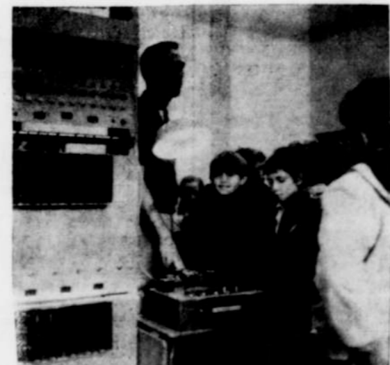
Buck Hicks, Valley Telephones Central office repair man, shows students the repair equipment for Central office equipment.
