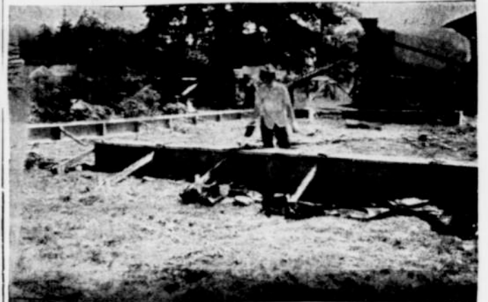
In the above picture in the foreground, Mrs. Gale Dorothy, local teacher, can be seen swinging a trowel smoothing out the cement on the foundation of the barn they are building. Gale was laid off by the carpenters strike. Maybe Mrs. Dorothy is enjoying some "woman's lib," but that is doubtful. Jerry Pittam is responsible for the photo.
