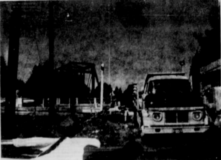
The above picture shows the men, trucks and equipment on hand to repair the bridge on First street, heavily damaged when the Southern Pacific freight train and a logging truck hit, throwing the logs on a car occupied by Mrs. Carl Kelly. The accident occurred in June and the crews have been working the past week on the repairs.—Mill City Enterprise photo.
