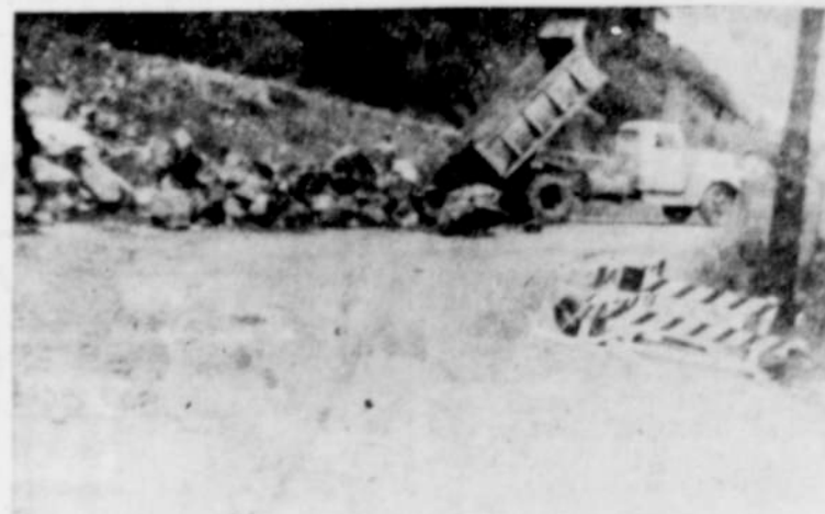
The old approach to Mill City is no more. This shot was taken as the dump truck unloaded a pile of rock sealing this approach, which has long been deemed a hazard in Mill City. This hill has a record of many wrecks, some of them landing right through the front door of the Mill City Tavern.
