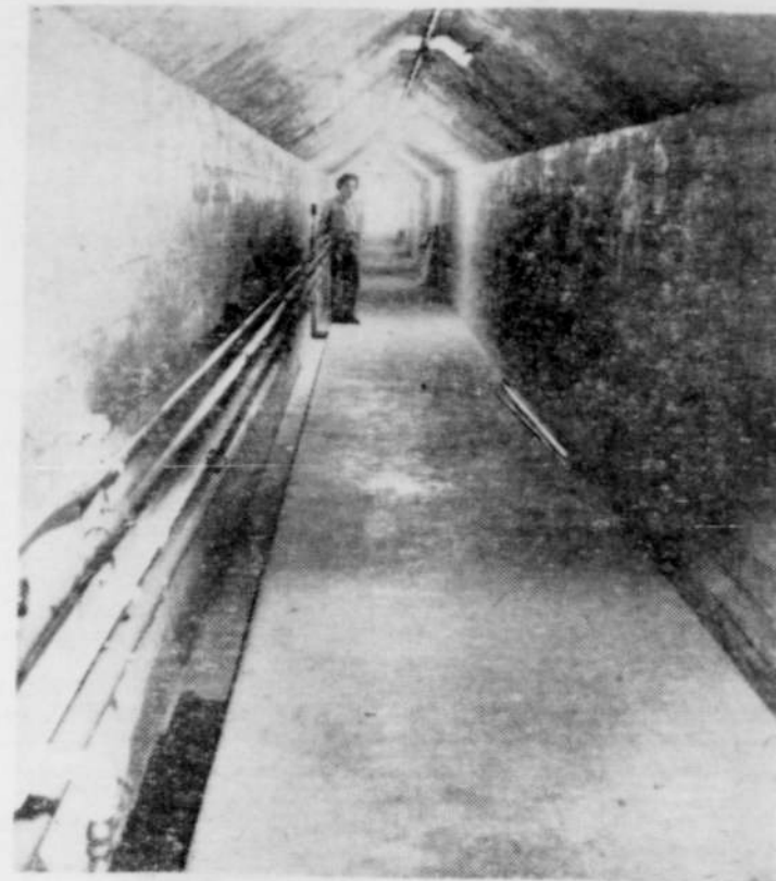
Sound of the North Santiam River pounding through Detroit Dam can be heard from this tunnel, one of many that catcomb interior of the project. Picture was taken near base of dam and shows all but 20 feet of the dam's width at this point. (Photo courtesy The Statesman)
