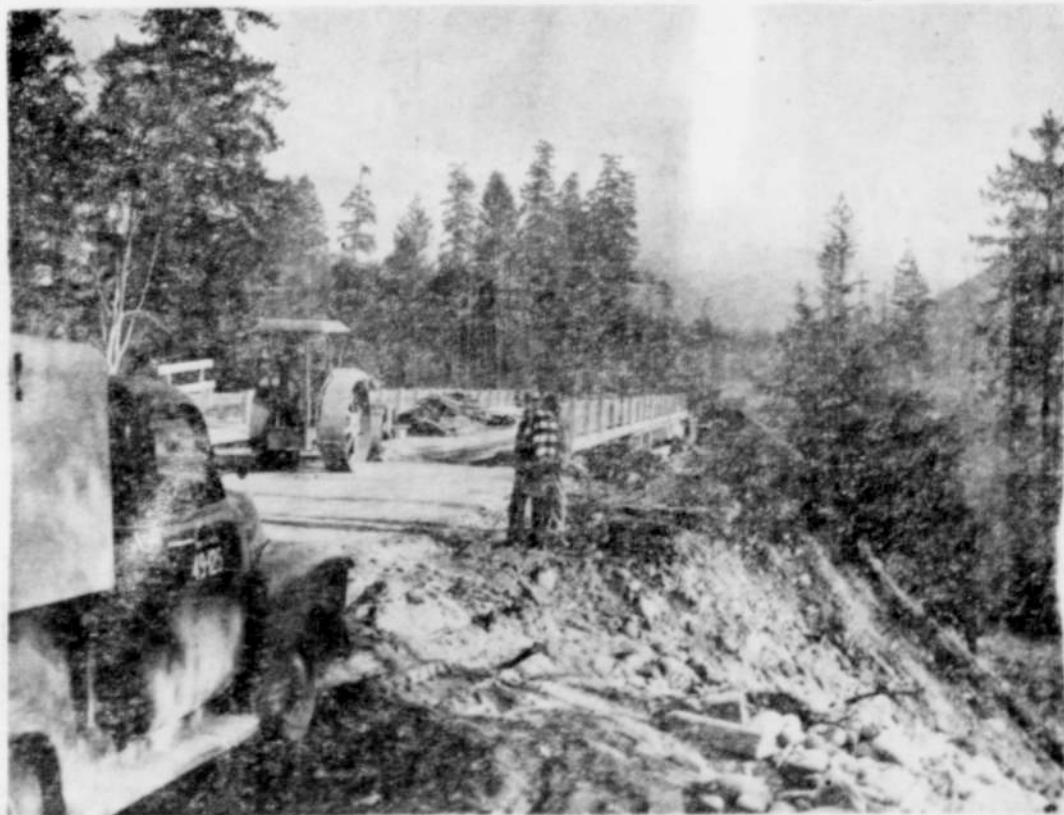
Work was progressing rapidly two weeks ago on the new North Santiam bridge when this picture was taken. This was the last link in the new highway from Mehama to Mill City on the Marion county side of the river. Last week the state highway commission opened the new bridge to public travel. (Photo courtesy The Oregonian)
