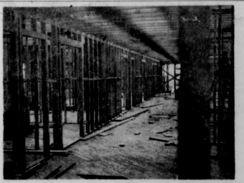
The interior of the main ward of the Santiam Memorial hospital is at this stage of construction, with electrical work, plumbing and steam fittings roughed in. Today, according to R. L. Martin, contractor, workmen are laying the face brick, setting the window frames on this ward and putting on the roof. The maternity ward is also well along and the entire job going so well that it is expected to be completed by Christmas. (Stayton Mail Photo)
