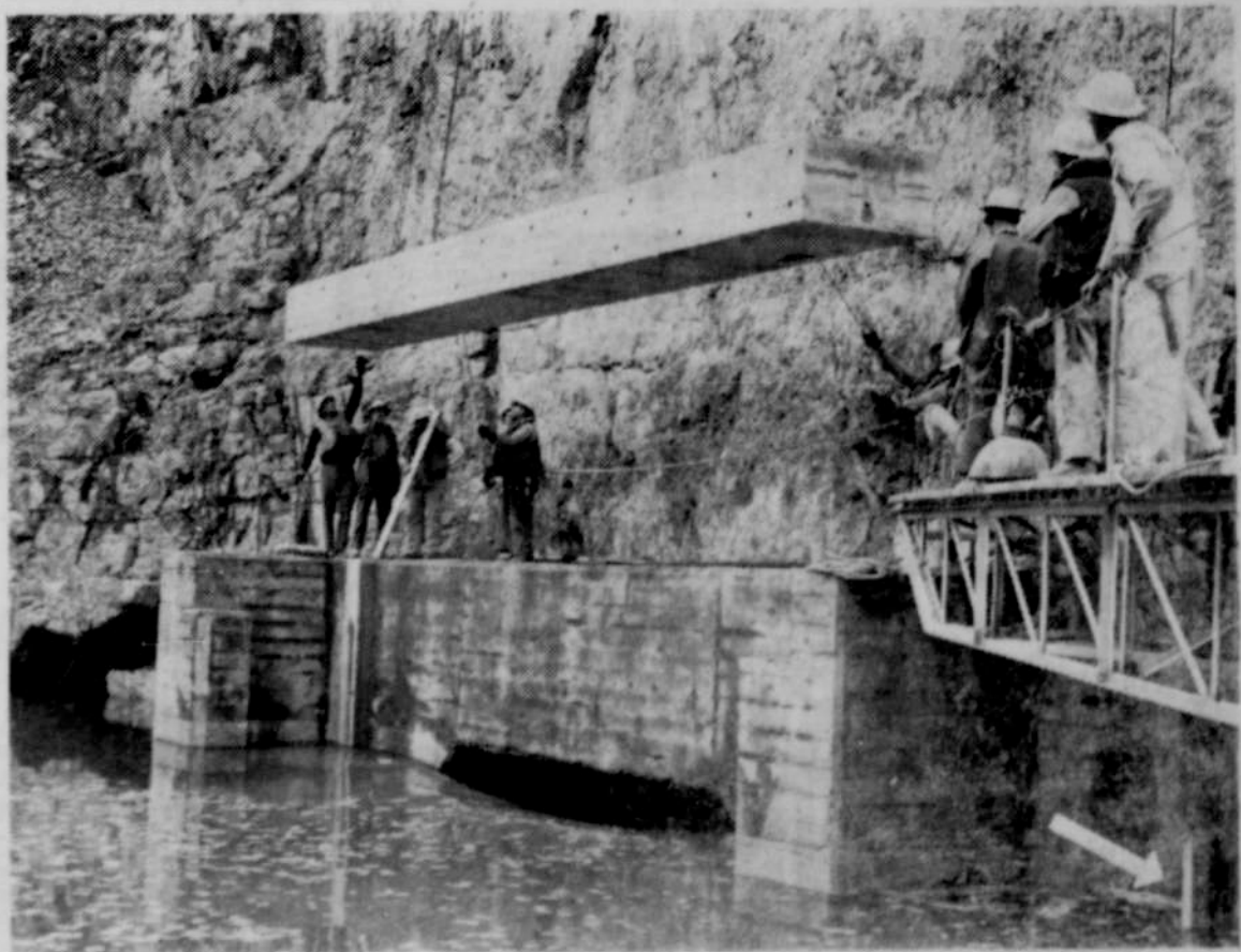
Next to the last concrete "log" goes into position at the mouth of Detroit dam diversion tunnel. The crane operator stationed many feet above these CBI workmen lowered the massive re-enforced concrete slabs into place Tuesday morning. Arrow points to the small by-pass tunnel which kept water flowing in the North Santiam river below the dam during the early filling up stage of Detroit lake. Eventually the North Santiam river will form an eight and one-half mile long reservoir above the dam. (Photo courtesy of Robert Veness and The Capital Journal)
