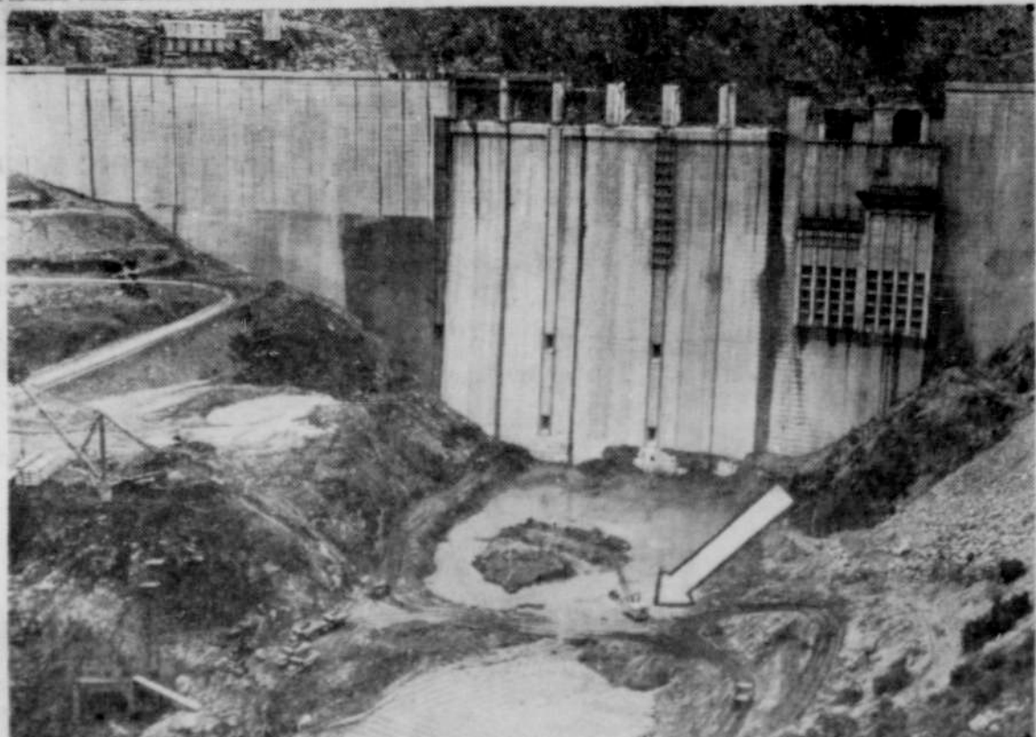
Detroit Dam, now 100 percent complete, dwarfs a CBI crane engaged in clean-up operations on the bed-rock of the North Santiam river immediately in front of the up-stream face of the dam. Arrow points to crane. Tuesday was the last day such a picture as this could be taken. Detroit Lake is now rising. The North Santiam river at Mill City is flowing at a very low stage. (Photo courtesy of The Capital Journal)
