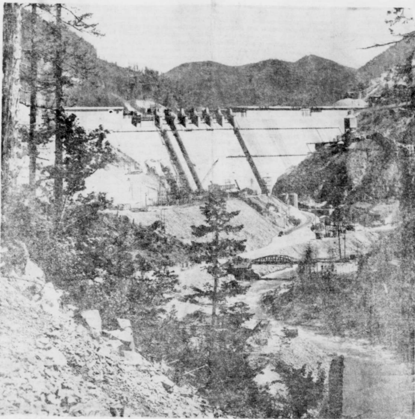
Detroit dam, nearing completion, towers over the North Santiam River Canyon, ready to serve as flood controller and power producer. Engineers expect to block the diversion tunnel this week to start water backing up in a huge man-made lake. Water stored behind the dam will serve a three-fold purpose—to turn the generators which will produce electricity for Willamette valley cities, to keep the Santiam and Willamette rivers from flooding rich farm lands in flood season, and to form an extensive
