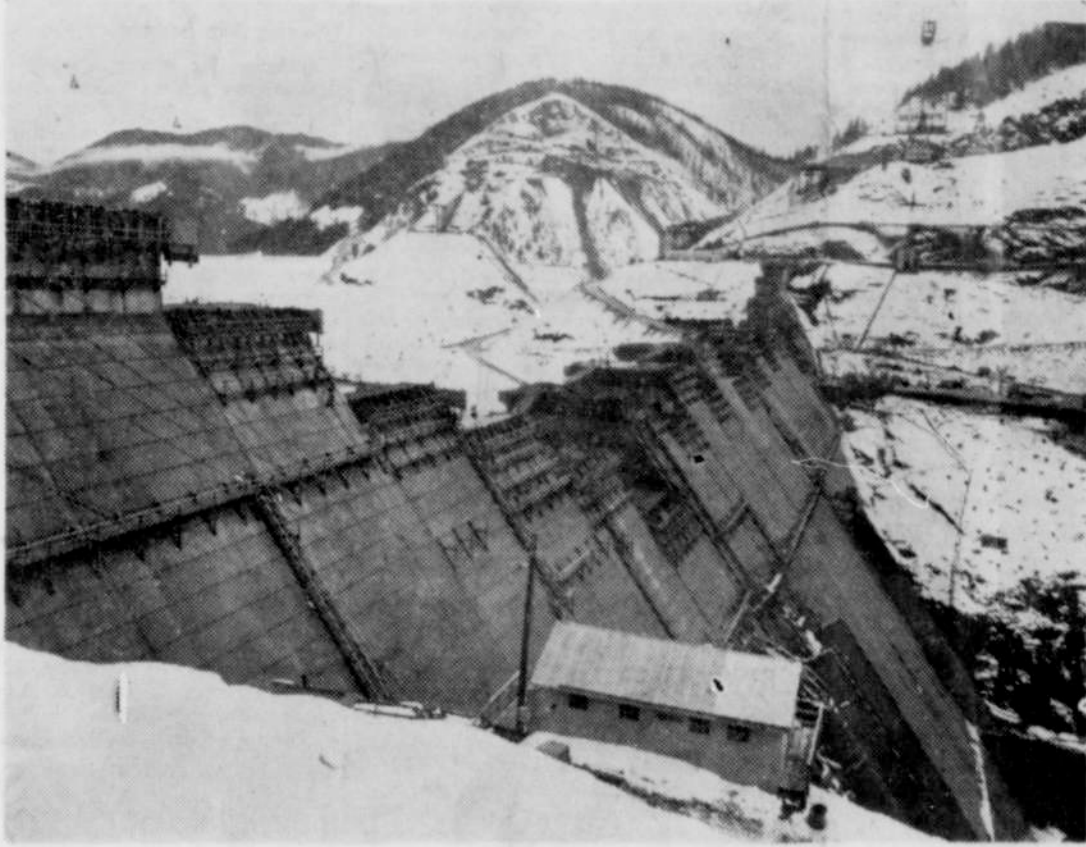
This recent view of Detroit dam shows its rapid rise to its projected height of 463 feet. The dam is 1580 feet long and 335 feet at the base, and when completed will contain one and one-half million cubic yards of concrete and seven million pounds of steel. Consolidated Builders, Inc., contractors on the project have only lost a few days operation due to weather. The dam project is scheduled for completion in 1953 with the estimated cost of the entire project set at $70,000,000. (Photo courtesy of Robert Veness and Capital Journal)
