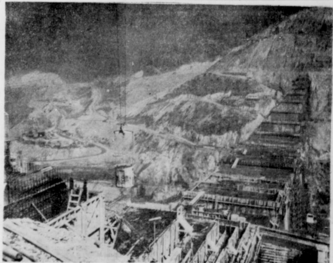
It is becoming increasingly clear that Detroit dam is well along on the construction road. Latest reports show that Detroit dam concrete pouring is 66 percent complete. This means that 66 percent of 1,400,000 cubic yards of concrete have been poured. Detroit dam is a flood control and power dam, part of the corps of engineers' Willamette Valley project. One of the huge "mud-buckets" in use on Detroit dam may be seen hovering above a concrete section in this view of the dam. The bucket is carried the entire length of the construction work along a cableway strung across the North Santiam river chasm. The operation of this unique cable-pulley set-up is the major attraction for sight-seers. (Photo courtesy of Capital Journal)
