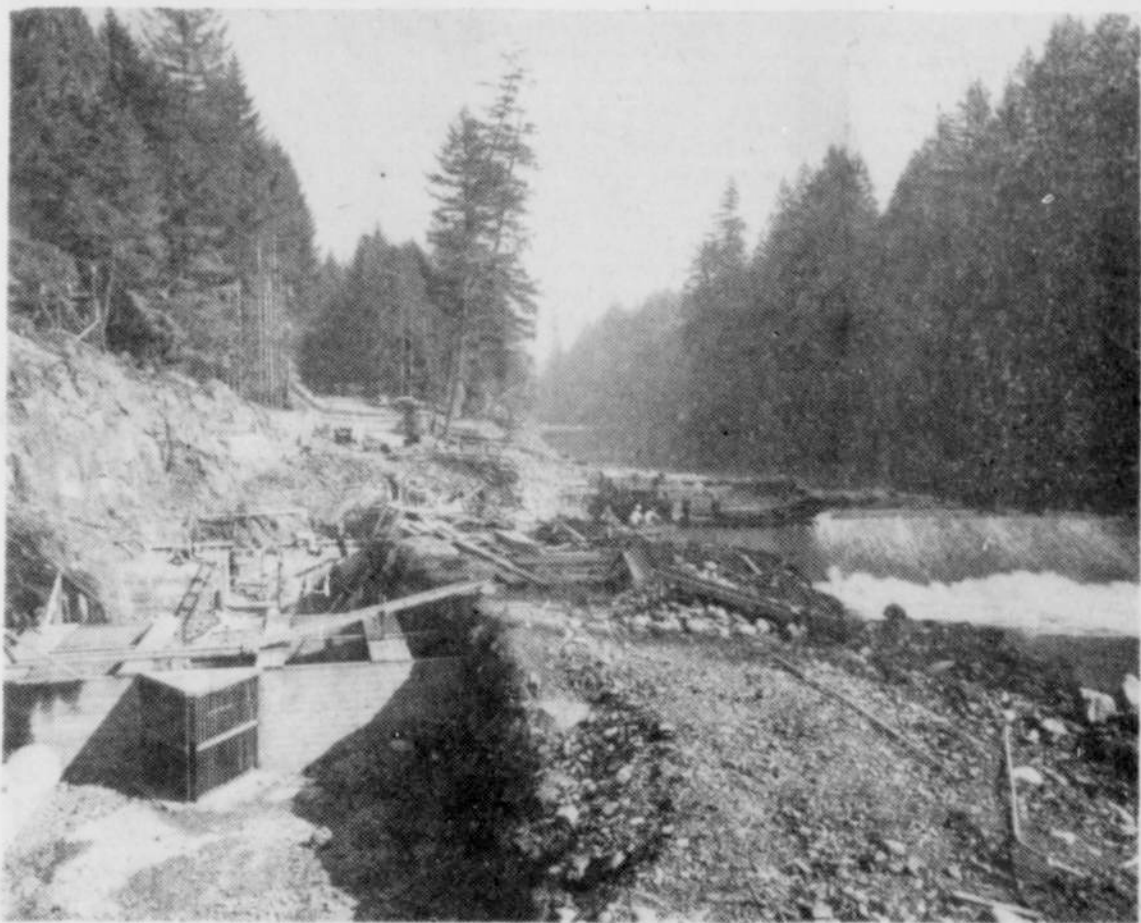
Lee Hoffman, contractor for the Corps of Engineers, will soon complete construction of the Minto egg-taking station located near Gates. This interesting facility makes possible the taking of eggs from salmon in the North Santiam river. Although this project, consisting of a 182-foot long dam across the river and a series of fishways and holding ponds, is being constructed by the federal government it will be turned over to the state of Oregon. Salmon eggs taken at Minto station will be transported to Marion Forks fish hatchery. The Minto station dam is 12 feet high. Phil Callender, foreman for Hoffman, stated that a recent flash flood ripped out one concrete retaining wall. Construction work on the Minto station probably will be complete next month. The holding pond maze can be seen to the left in the picture. The river itself can be seen sliding over the Minto station dam to the right. (Photo courtesy of the Capital Journal)
