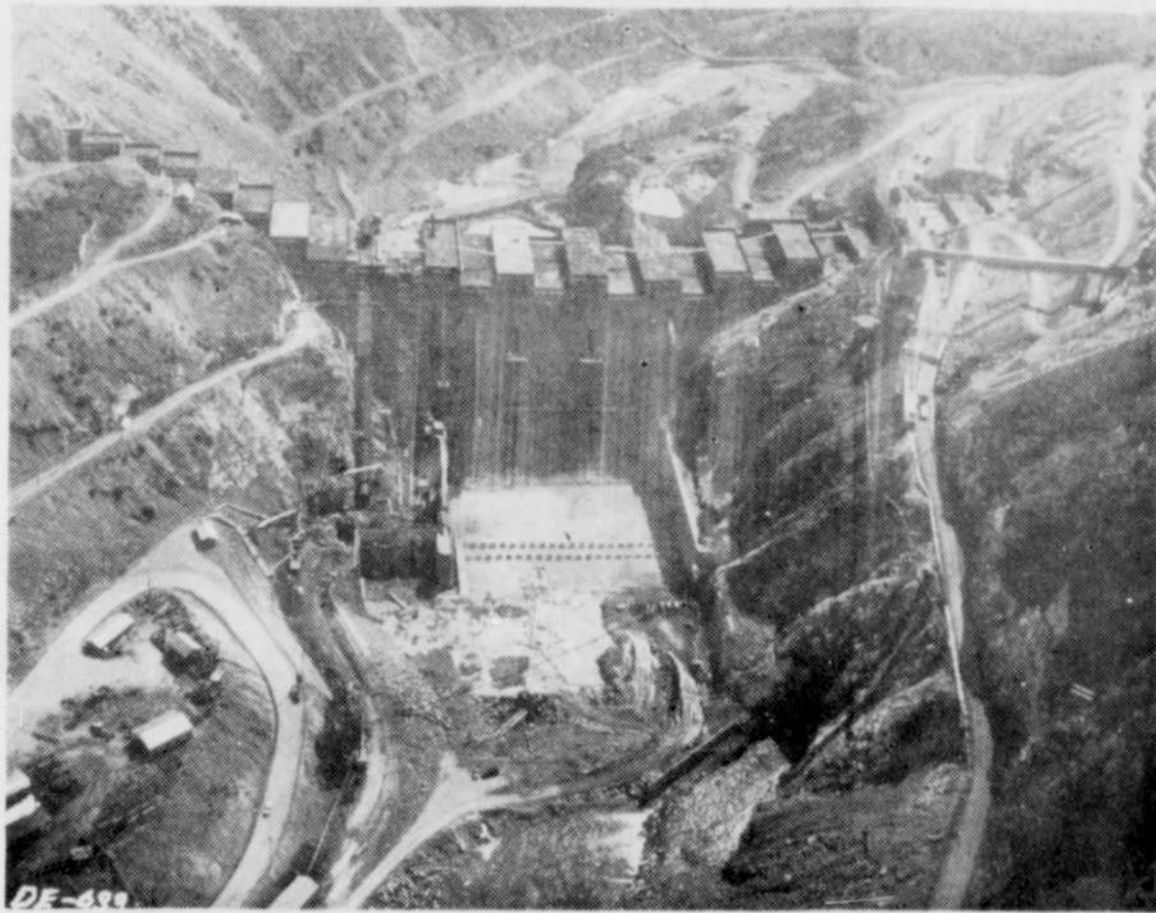
The Corps of Engineers felt that the progress of Detroit dam warranted their taking a photo of it also—so here is the result—an excellent aerial photo of the down-stream face of the massive Detroit dam. Concrete baffle walls may be seen in the center of the picture in the very bottom of the North Santiam river bed. The purpose of these baffles is the breaking up of the headlong rush of the waters which will cascade downward from time to time. The diversion tunnel is at lower right near the fork of the road in the river bottom. (Photo courtesy of the Capital Journal)
