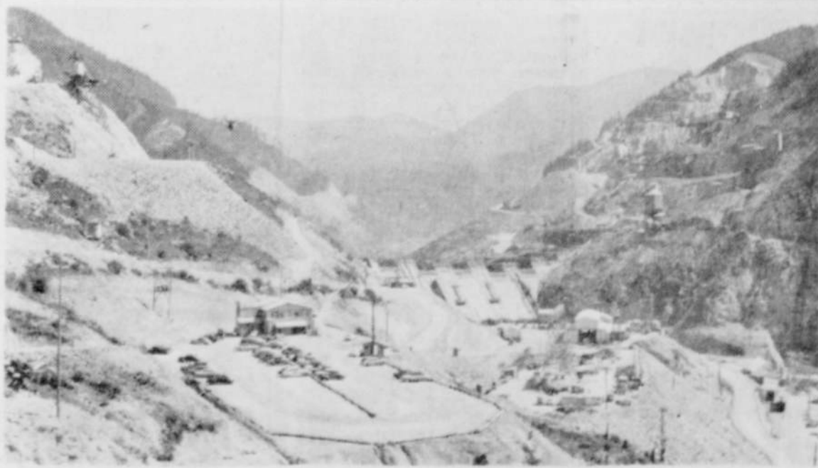
Another down-stream picture of Detroit dam is reproduced above. This photo was taken from a vantage point below the level of the North Santiam canyon highway. The parking lot shown to the left of the dam is for CBI personnel and employes. The huge dam is gradually rising higher and higher until finally it reaches the level of the canyon highway. Some 70% of the concrete going into Detroit dam has been poured. (Photo courtesy of the Capital Journal and Robert Veness)
